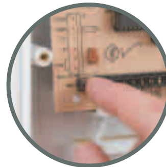
Walk / Alarm Test
